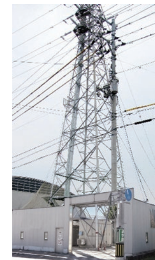
66 kV transmission tower
