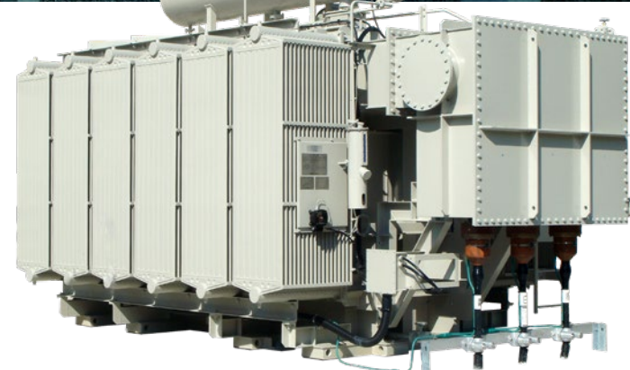
66 kV class oil-immersed transformer
