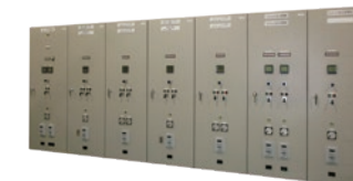
High voltage switchgear
