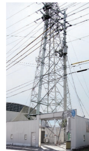
66 kV transmission tower
