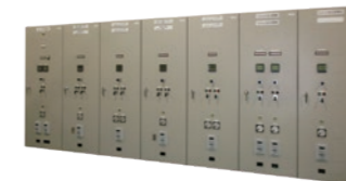
High voltage switchgear
