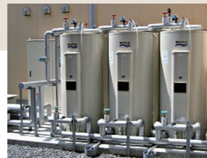
Commercial parallel hot water supply system
