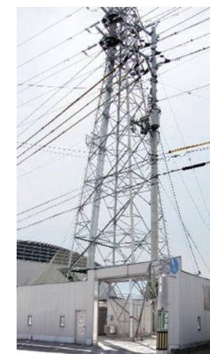
66 kV transmission tower
