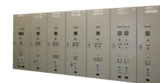
High voltage switchgear
